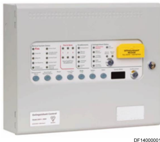
Figure 3-38 Extinguishant control panel
